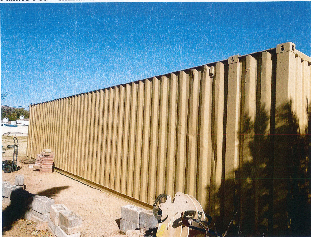
Painted Pod – replaced rotted storage from previous owner
