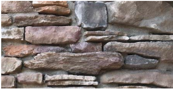
EXISTING Stonework--- LRV 24
