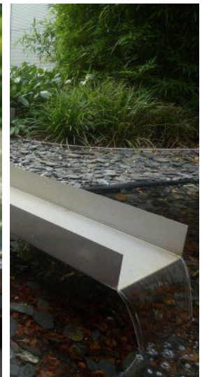
Disconnecting a downspout allows rainwater to supplement irrigation in the landscapes.
