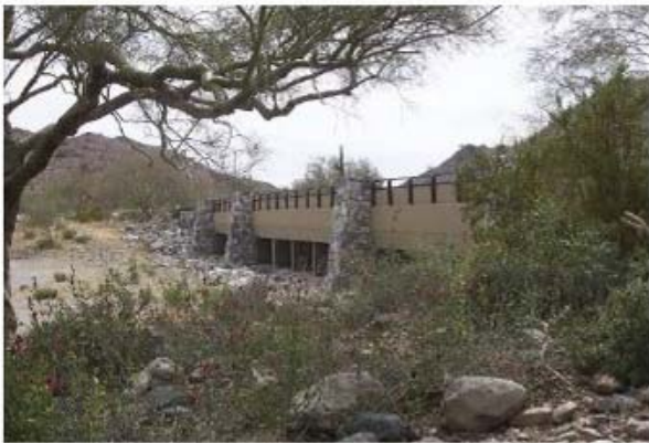
Example of Box Culvert Bridge. Wash Crossing in Parcel B to be Similar in Design.
