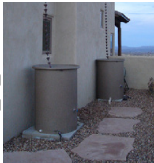
Cisterns can store rainwater to be re-used for future landscape irrigation.
