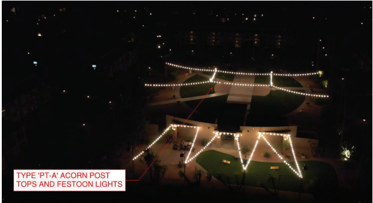
Post top “acorn” lights and festoon lights illuminate the event lawn with soft uniform lighting. Besides the tennis courts, this is the brightest area on site. Note that there are additional floodlights mounted on palm trees for additional event lighting that were not energized in this photo.
