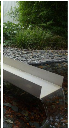
Disconnecting a downspout allows rainwater to supplement irrigation in the landscapes.
