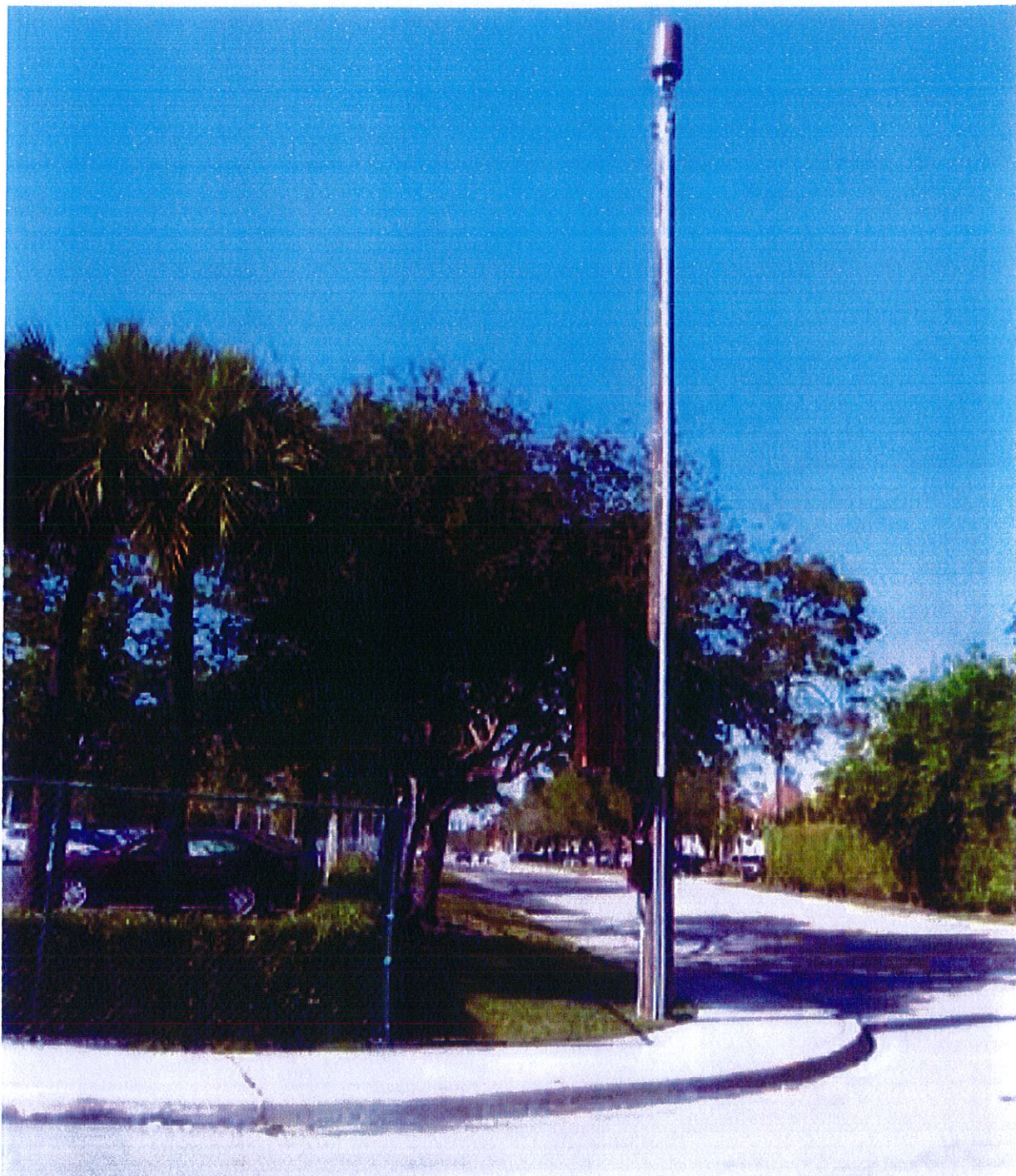
Figure 3. Crown Castle pole-based small facility deployment in Broward County, Florida. 3
