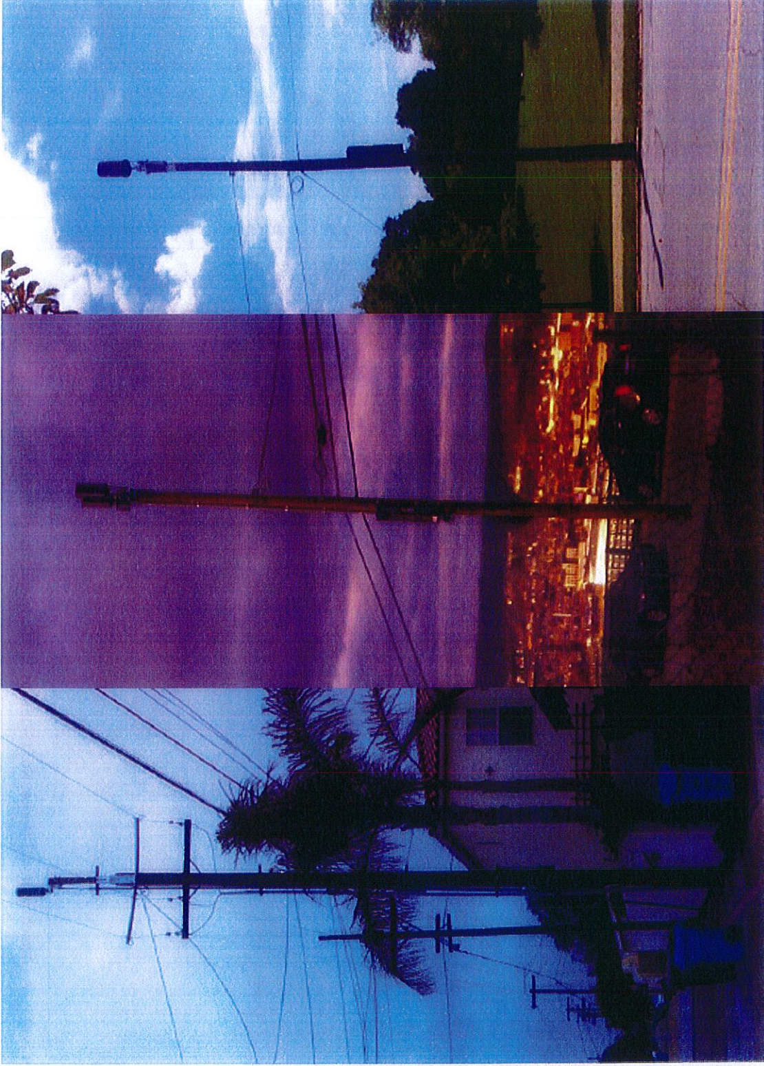
Figure 11. Typical Crown Castle small facility deployments on utility poles 11
