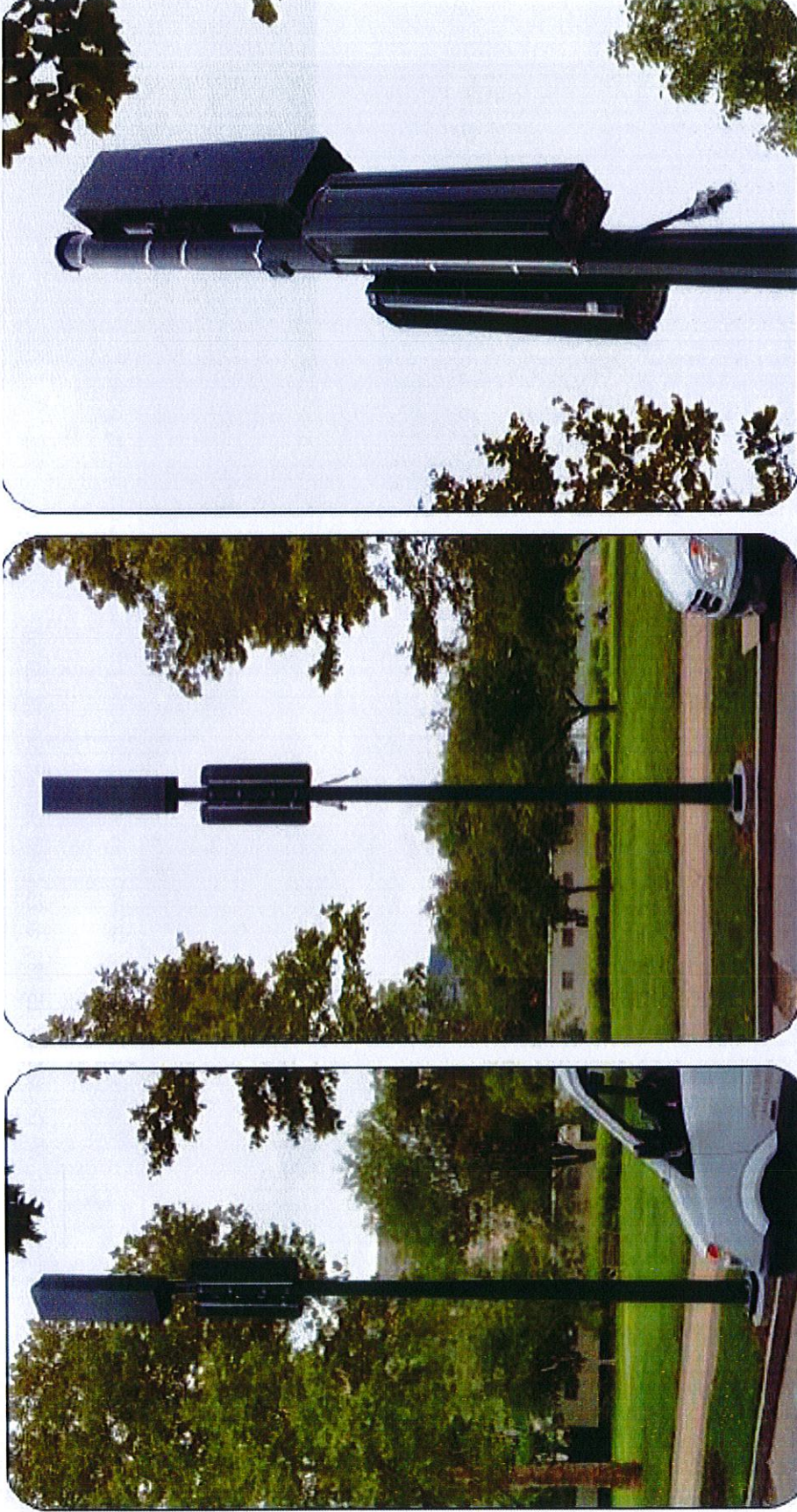
Figure 12. Crown Castle multi-carrier pole-mounted small facility deployment 12
