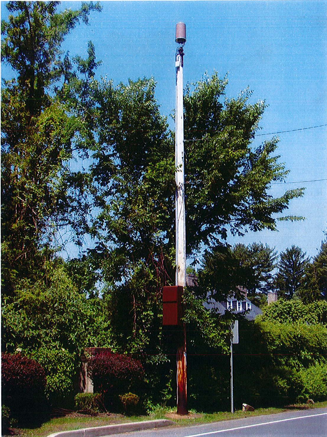
Figure 2. Crown Castle small facility deployment on a utility pole in Princeton, NJ. 2
