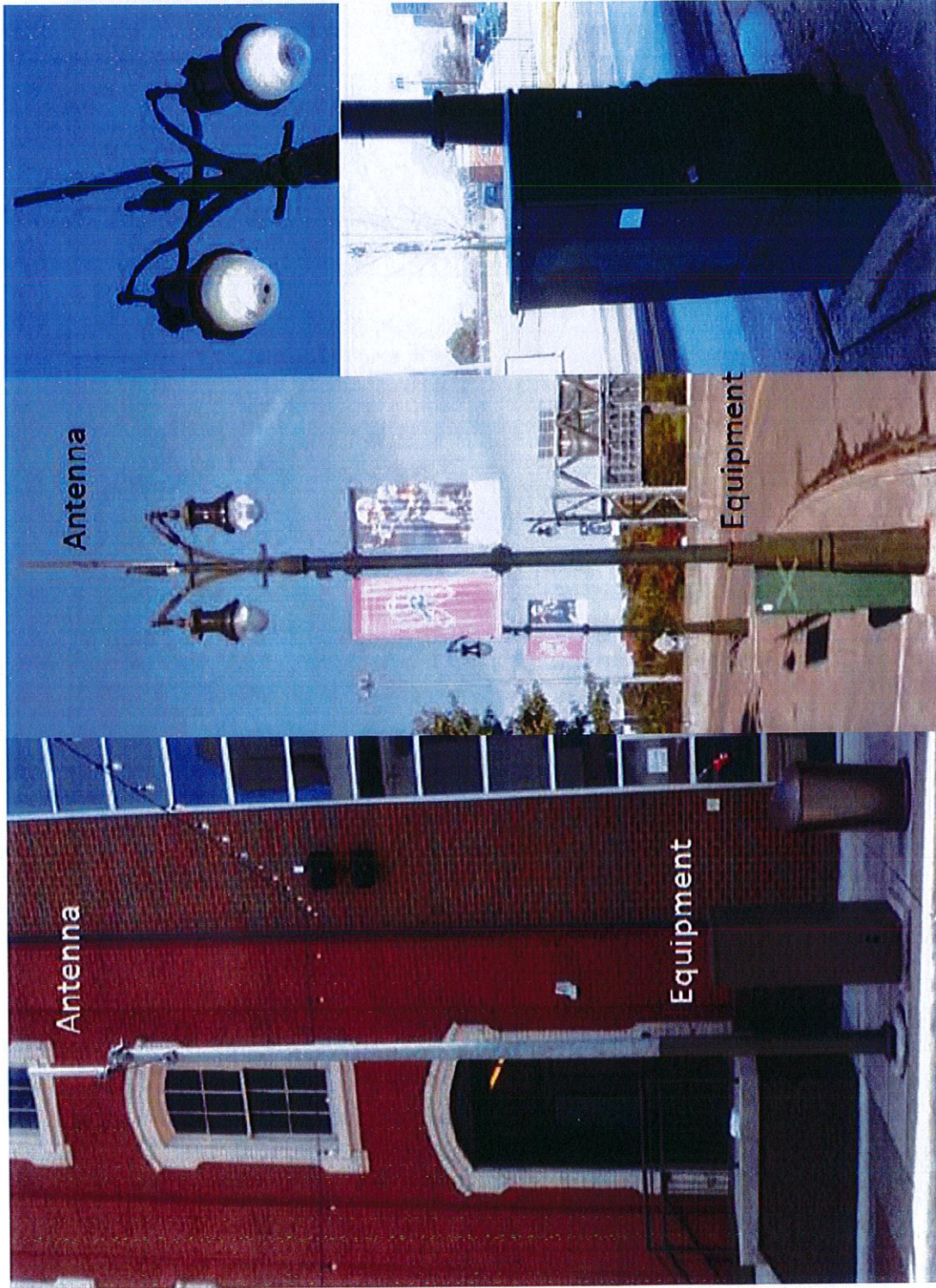
Figure 10. Sprint small cell deployments in Detroit 10
