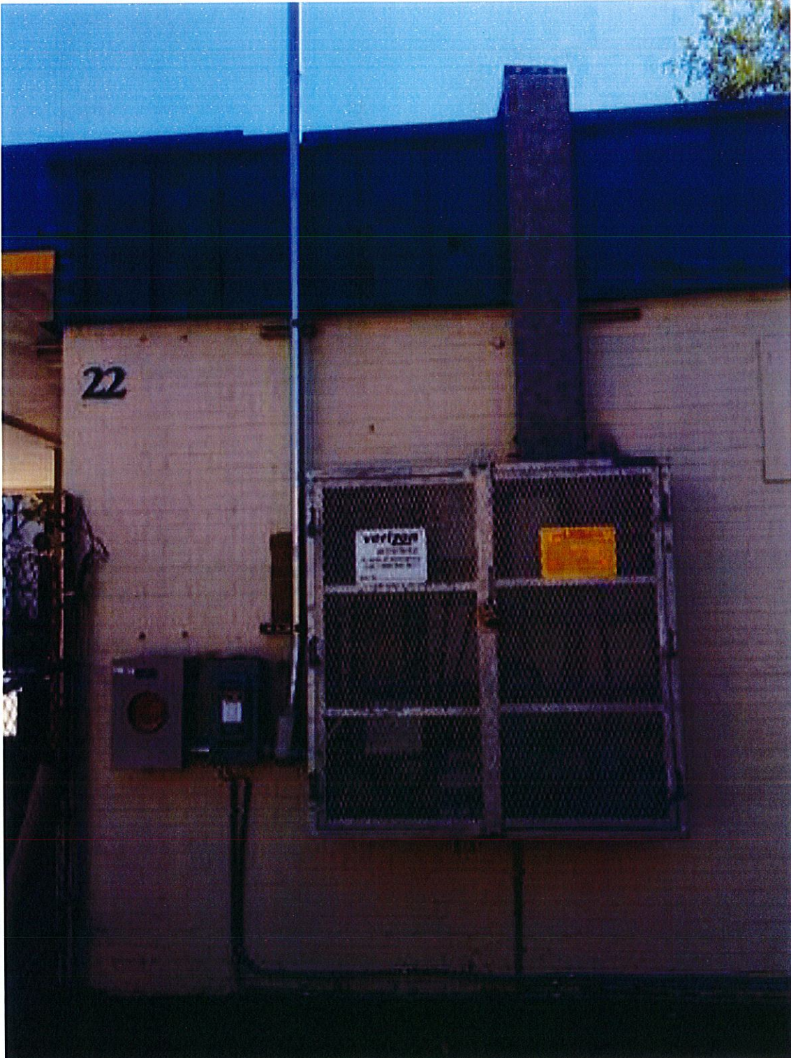
Figure 8. Wall-mounted Verizon small facility deployment. 8
