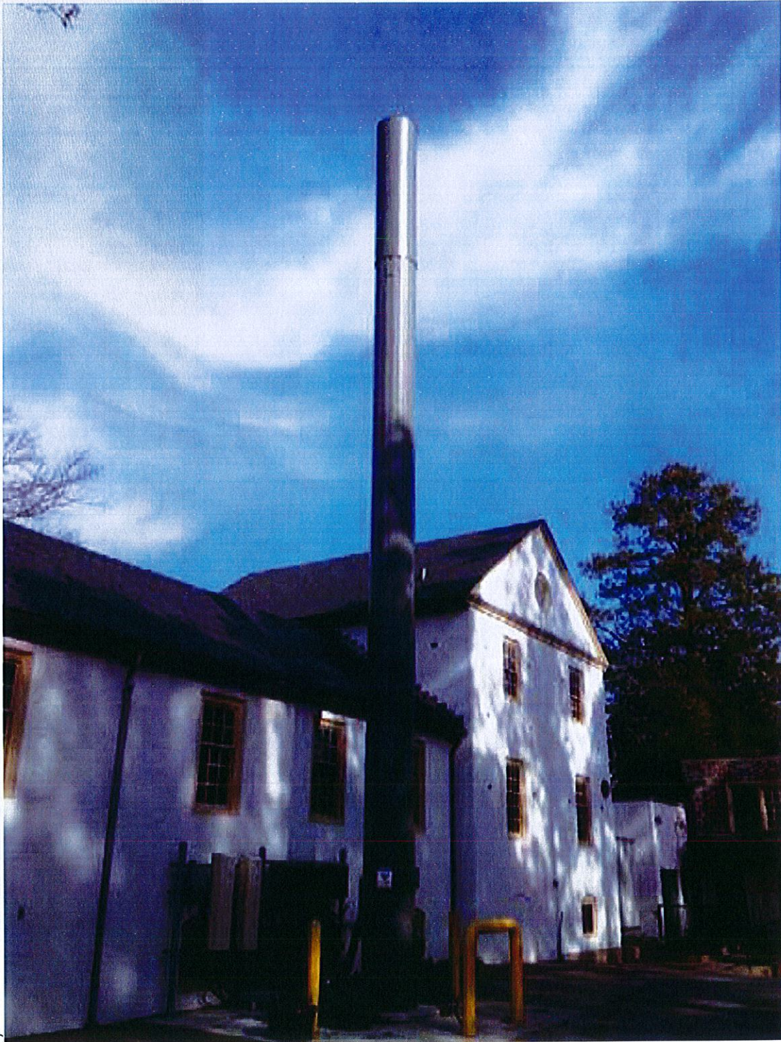
Figure 15. Crown Castle small facility deployment at the Williamsburg Inn in Colonial Williamsburg. 15
