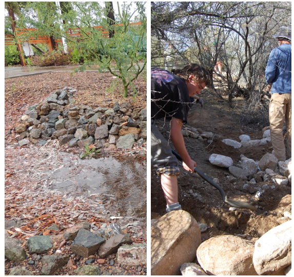
Vegetated swales accept stormwater for conveyance, storage and infiltration.
