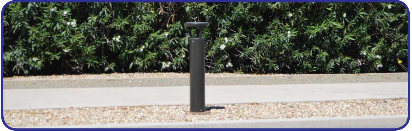
Figure 2.8: Solar Lighting Bollard
