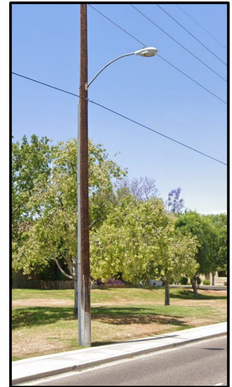
● - Overhead electric pole
