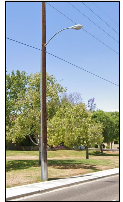
● - Overhead electric pole
